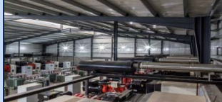
Heavy Fuel Oil Power Plant
